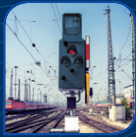
1 Trackside traffic control box Signal lights box
