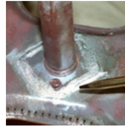
Pyro-Putty® 653 seals corroded burner manifold.
